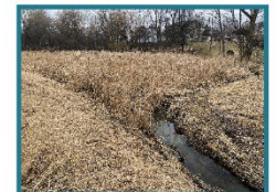
CC00231 5 Acre-Feet Detention Basin
